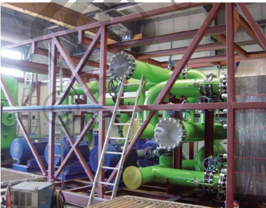
Figure 6. Pump container without roof and side walls
