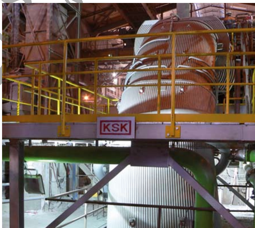
Figure 1. Off-gas bend connected to the EAF
