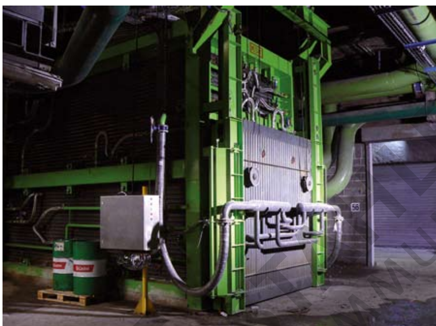
Figure 4. Lifting door at the face side of the combustion chamber
