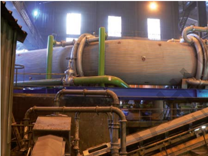
Figure 5. The hot gas duct is made up of five segments
